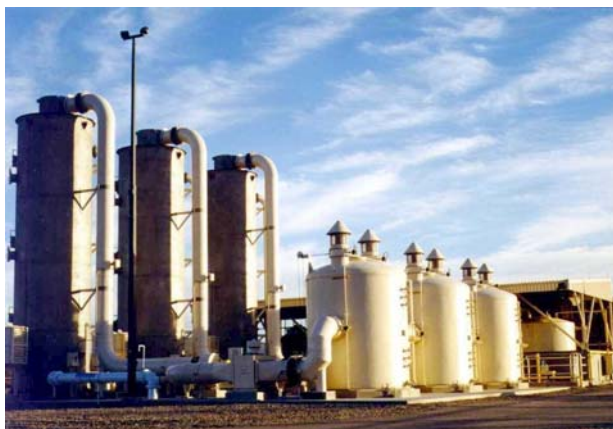
TARP Groundwater Treatment Plant
