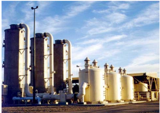
TARP Groundwater Treatment Plant
