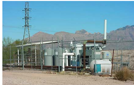
The City's Bioremediation and Soil Vapor Extraction System
