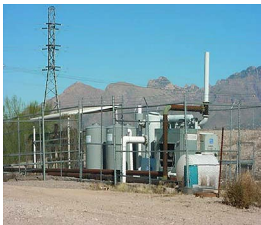
The COT's Bioremediation and Soil Vapor Extraction System
