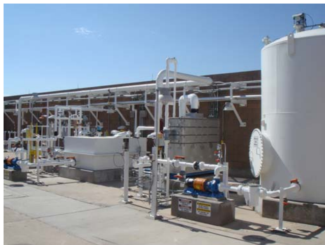
The Groundwater and SVE Treatment Plant at the Airport Property TIAA CERCLA Site
