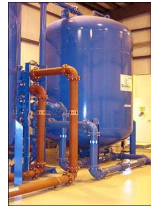
Carbon Chamber at EGTS
