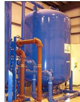
Carbon Chamber at EGTS
