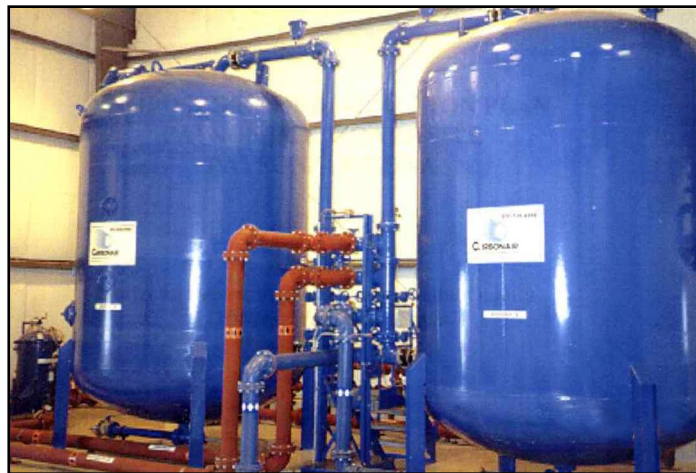
The Expanded Groundwater Treatment System (EGTS) Carbon Vessels.
