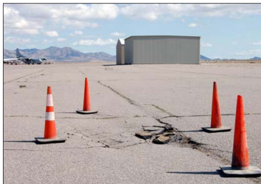
HMA Cap Failure
