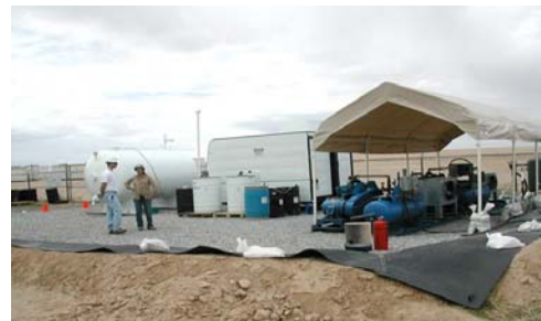
New Soil Vapor Extraction System
