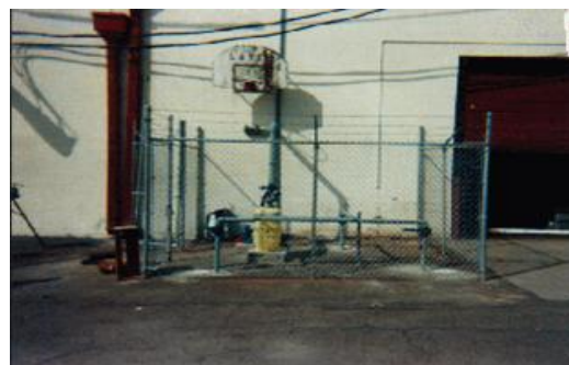
SVE System at Layke Facility
