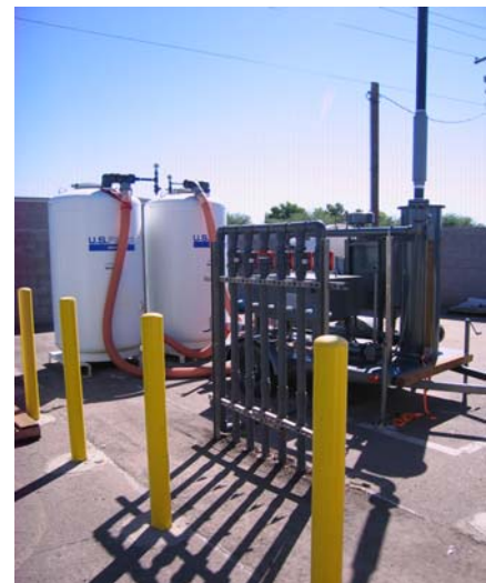
SVE Treatment System at Hill Brothers Chemical Company
