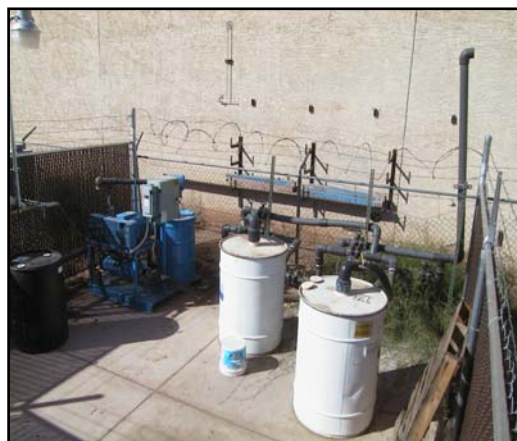
SVE System at WOC Facility
