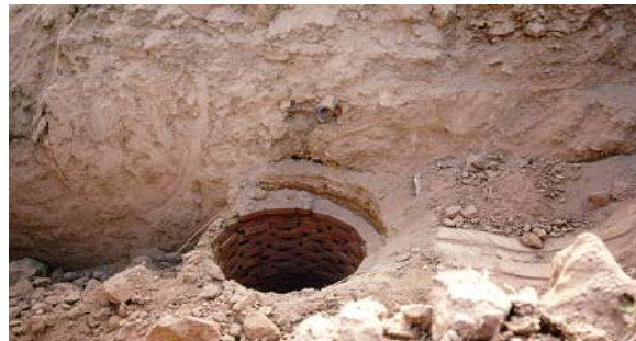
A Seepage Pit at WOC
