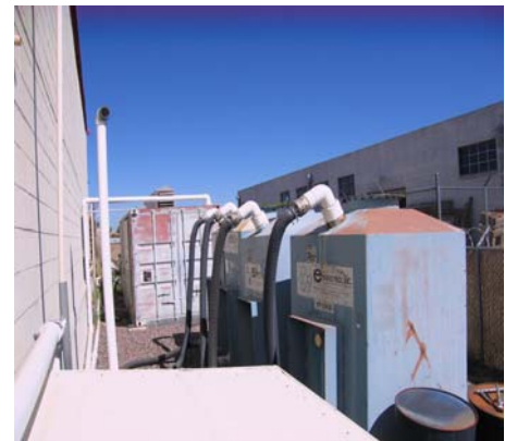
Soil Vapor Extraction System at VW&R facility
