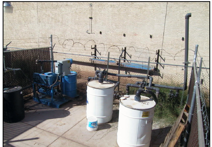
SVE System at the WOC Facility.
