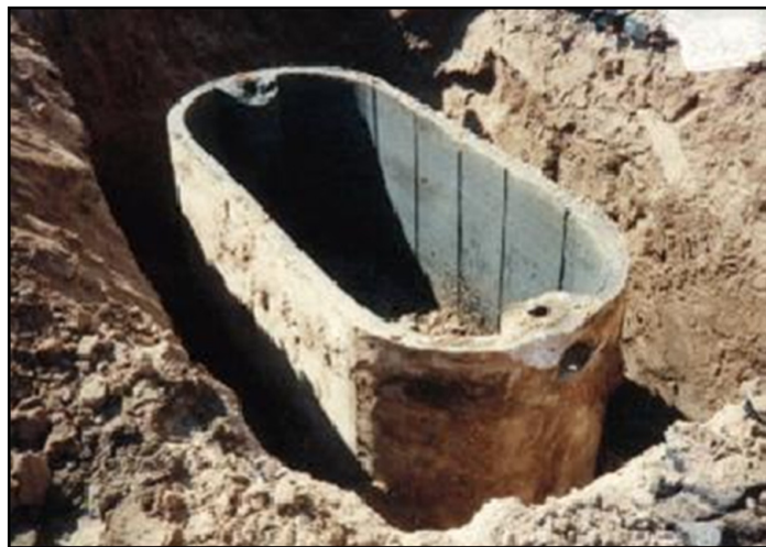
Underground Storage Tank at the Layke Facility.
