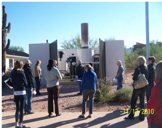
SVE System at ST035
