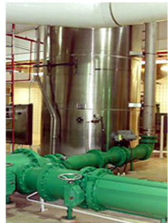
Inside one of the groundwater treatment facilities.
