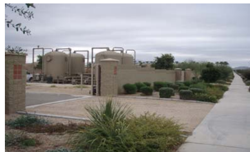
Well 33A Treatment System
