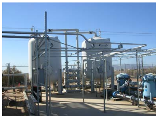
Main Treatment System
