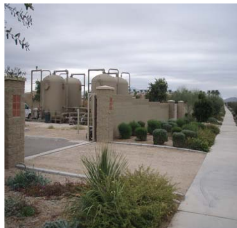
Well 33A Treatment System
