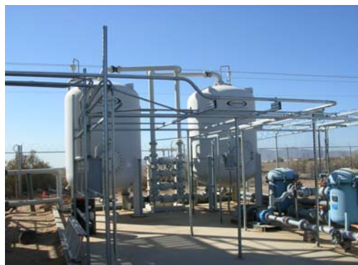
Main Treatment System
