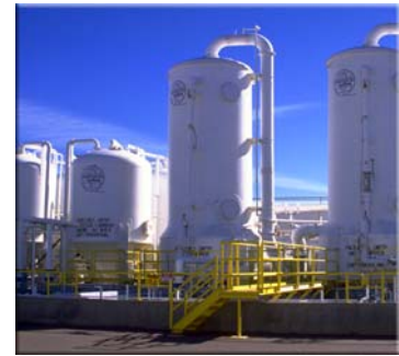
OU1 Treatment System 5005 E. McDowell Road
