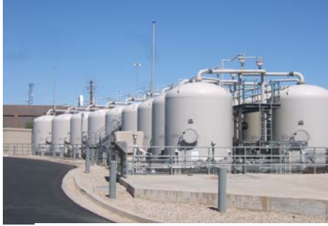
OU2 Treatment System 20 th Street & Washington Street
