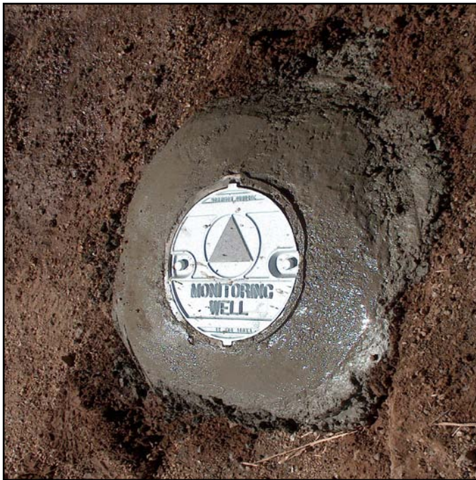
Finished Monitoring Well.
