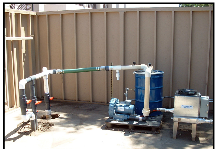
Soil Vapor Extraction (SVE) System.
